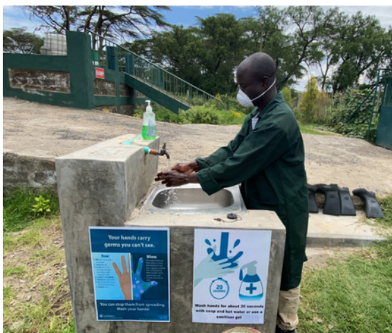
Handwashing station and signage at Sanivation's waste-to-resource facility in Naivasha, Kenya
